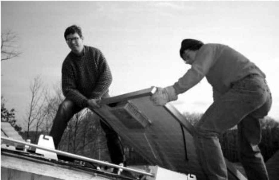
Figure 3. An installation of a SunSine 300™ ac photovoltaic module showing the fully integrated inverter mounted to the back surface of the photovoltaic module. The integrated connect cables run along the sides of the module.
