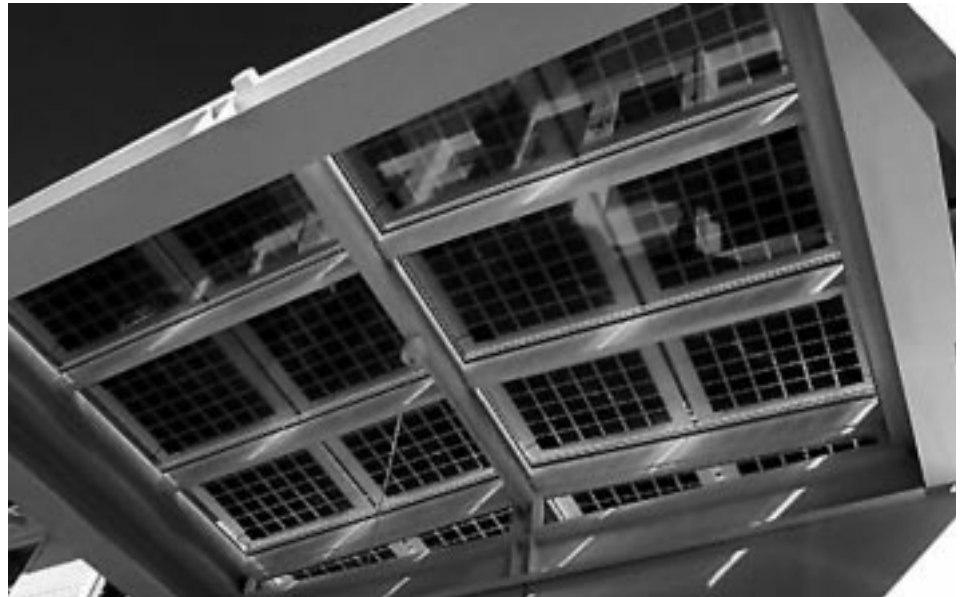
Figure 5. Building integration of photovoltaic systems relies on code compliance for installation.
