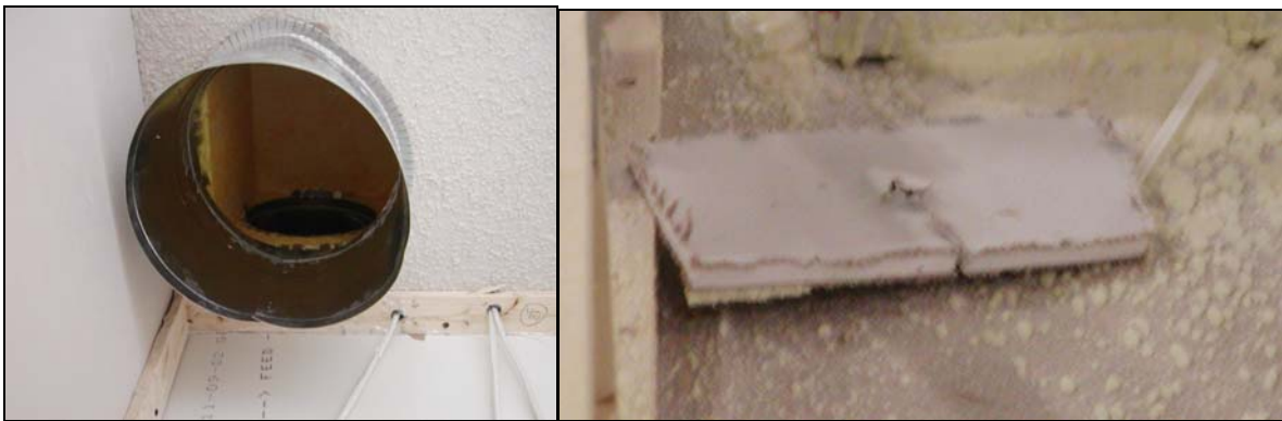
Figure 6 Left Holes cut free hand do not mate well with duct system components. Note round duct is jammed into an oval shaped cut out. Right Imprecise rectangular cutout for ceiling register creates poor joint.
