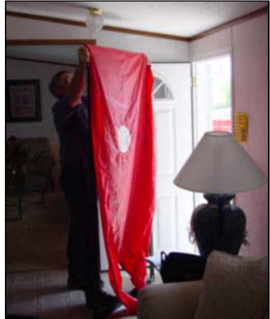
Figure 2 BAIHP Researcher Neil Moyer sets up blower door for testing the air tightness of a manufactured house.
