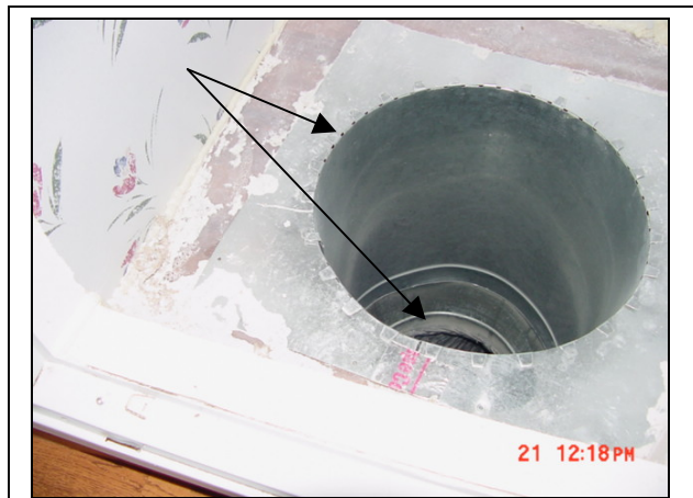
Figure 4 No mastic on return duct in plenum serving packaged heating and cooling unit. Mastic used elsewhere in the plenum and throughout house.
