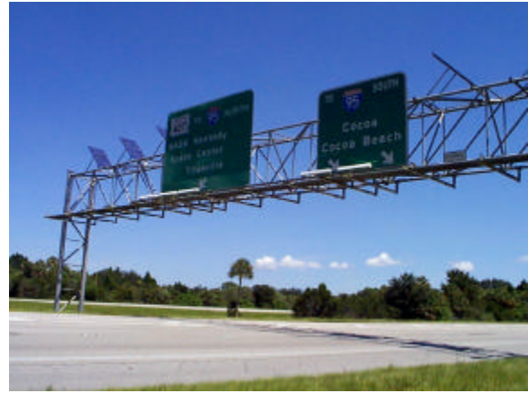
Figure 3-2. PV-powered highway guide sign lighting system.
