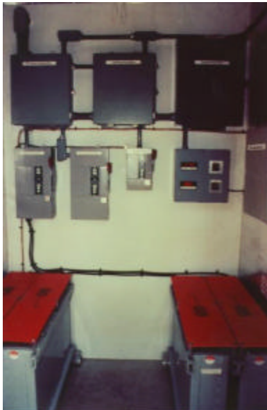
Figure 3-5. Guide sign lighting battery and control room.
