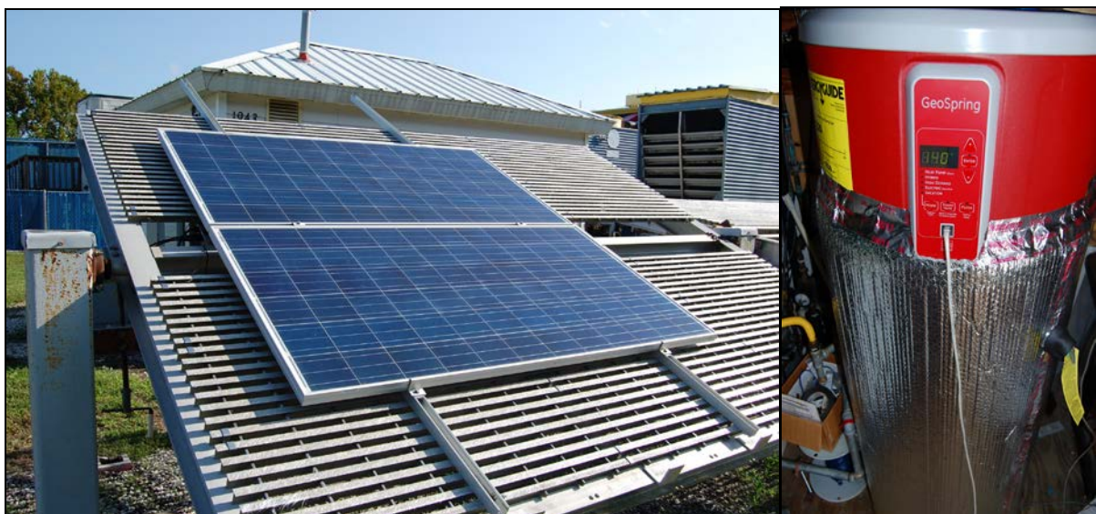
Figure 1: PV modules (310 Watts each) and 189-Liter HPWH shown with added insulation
