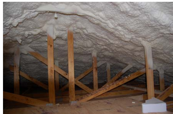
Figure 2: Roof deck insulation (R-27) featured on Builders Challenge Home in Rockledge, FL
