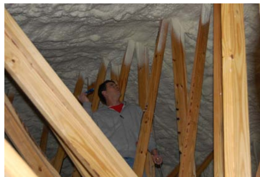
Figure 3: RH and temperatures were measured at peak and mid levels within the sealed attic.
