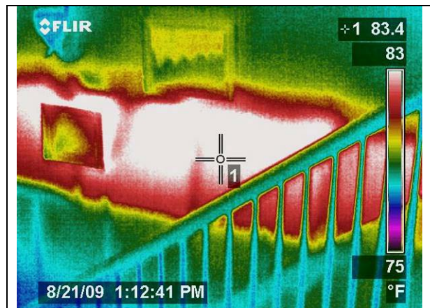
Figure 1 Infrared image shows that floor space behind wall is very warm. (Image credit C. Withers)
