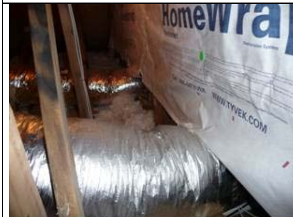
Figure 7 Open area of floor cavity below kneewall covered with house wrap on the west side of house.
