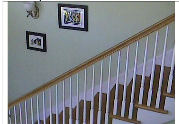
Figure 2 Photograph of IR image above. Floor space begins under the hung picture at top. (Withers)
