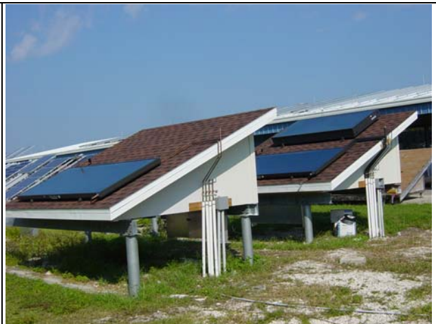
Figure 6. The solar collectors, with the ICS system in the rear top
