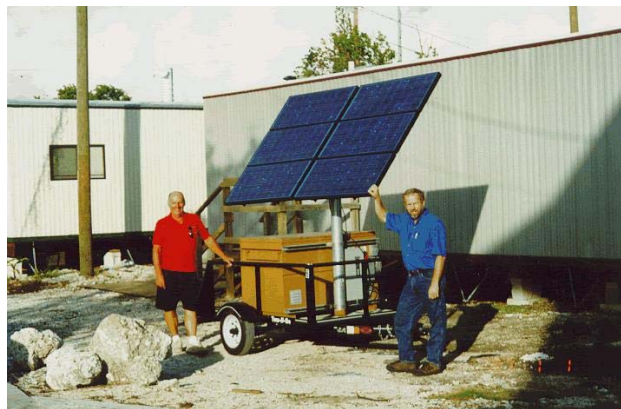
Figure 1: FEMA 500 Wp trailer
