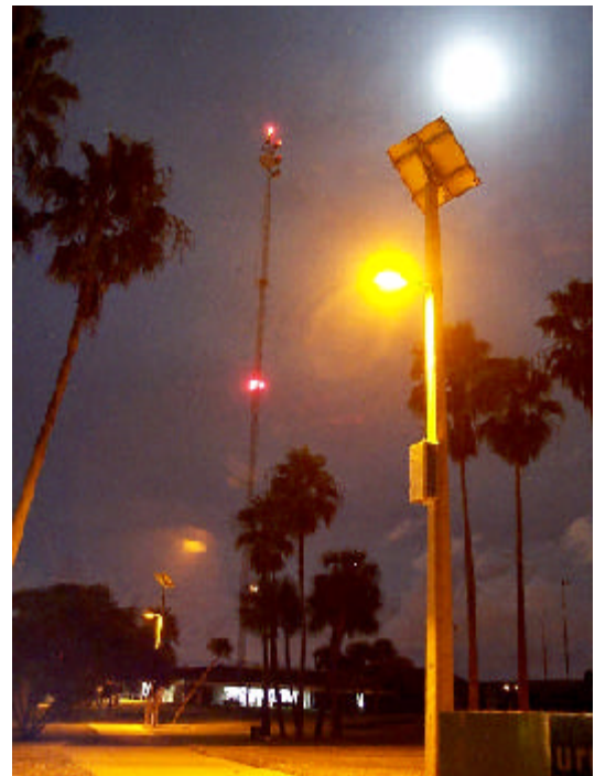
Figure 2. PV lighting system at night under full moon.
