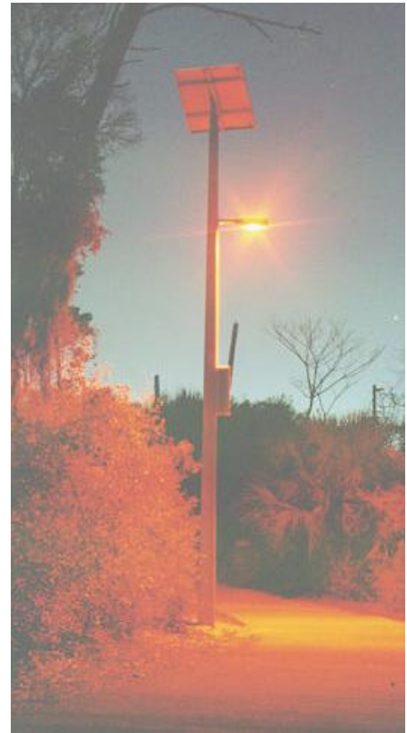
Figure 35. PV lighting system at night.
