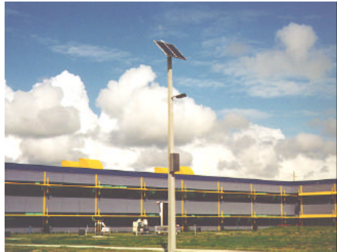
Figure 1. PV lighting system in front of FSEC building.
