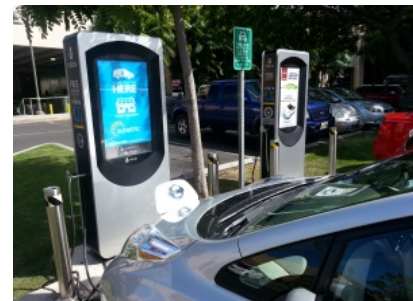
Figure 3. Hawaii Charging Station (photo K. McKenzie)
