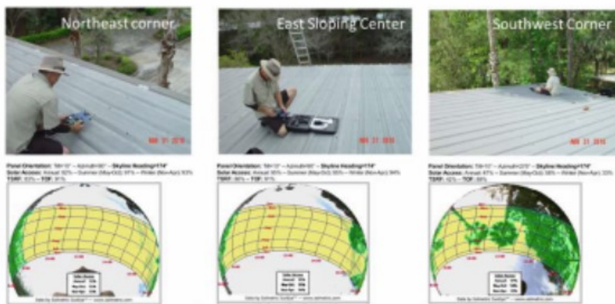
Figure 5: Roof line with skyline photo looking northeast (left), east (center), and shading at the southwestern corner (right) which is expected to be eliminated, enhancing solar access.
