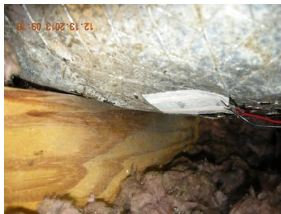
Figure 13. Moisture sensor strip adhered to bottom of ductwork
