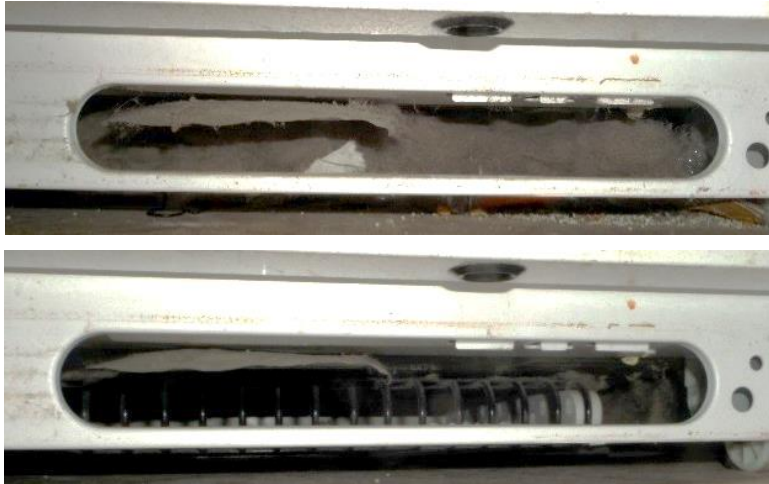
Figure 12. Site 54 - Refrigerator coils as found (top); Refrigerator coils cleaned (bottom)
