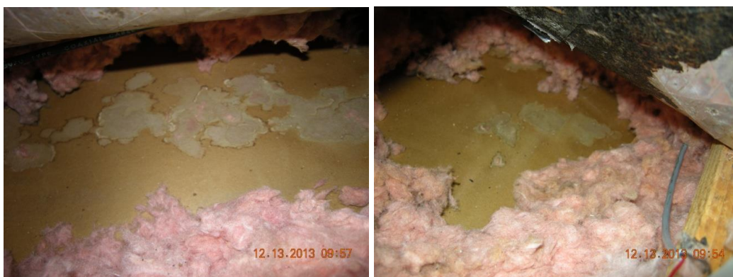
Figure 10. Historical moisture issues in attic under duct work
