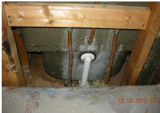
Figure 16. Missing air barrier behind tub
