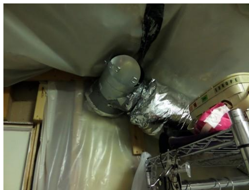
Figure 15. Second floor closet with shared supply ducting and open damper
