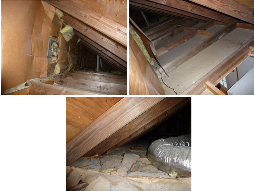
Figure 19. (a) Attic knee wall exposed kraft (top left), (b) Knee wall with cardboard covering exposed insulation (top right), and (c) Batt insulation with kraft paper exposed (bottom)
