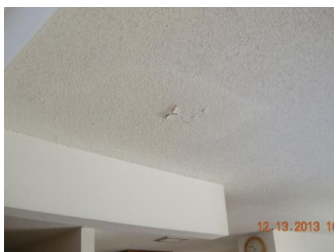
Figure 11. Ceiling damage close to room's supply duct
