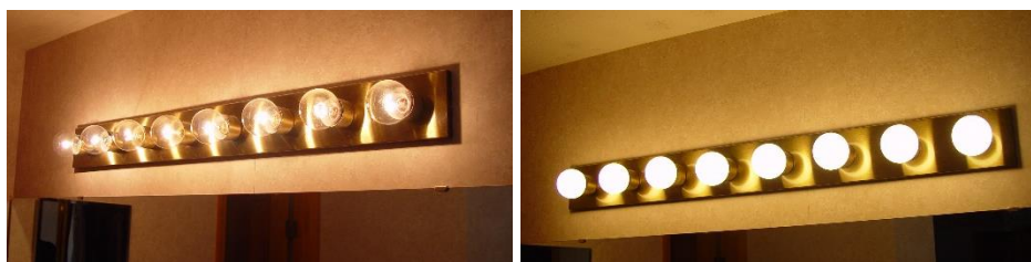
Figure 14. Site 7 - Eight-bulb retrofit from 360 watts of incandescent bulbs (left) to 72 watts of CFLs (right)
