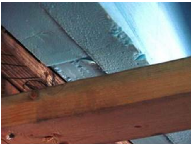
Figure 27. Joints of the first and second layers of blue board were staggered to further impede air flow.
