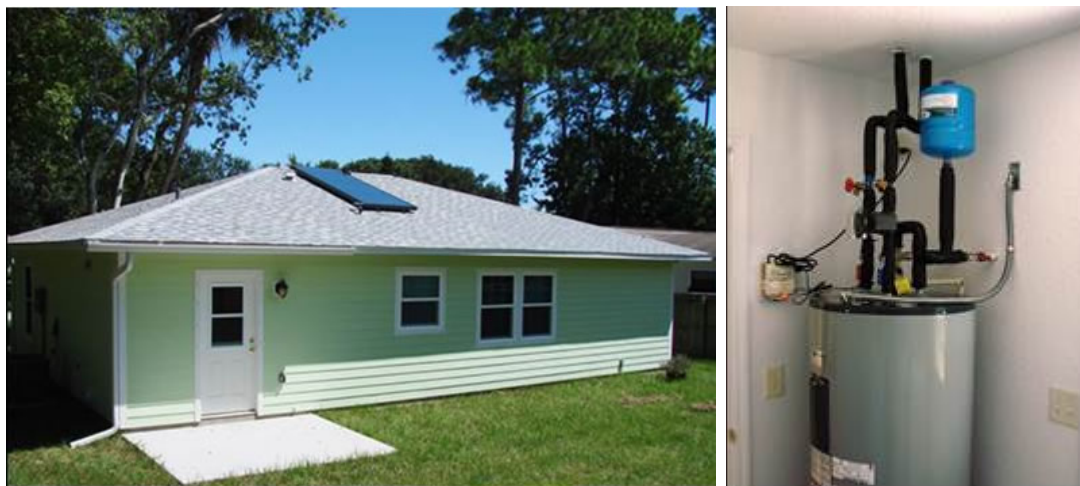
Figure 19. 40-ft 2 solar water heater installed on the south-facing roof (left) with an 80-gal tank in the utility room (right)
