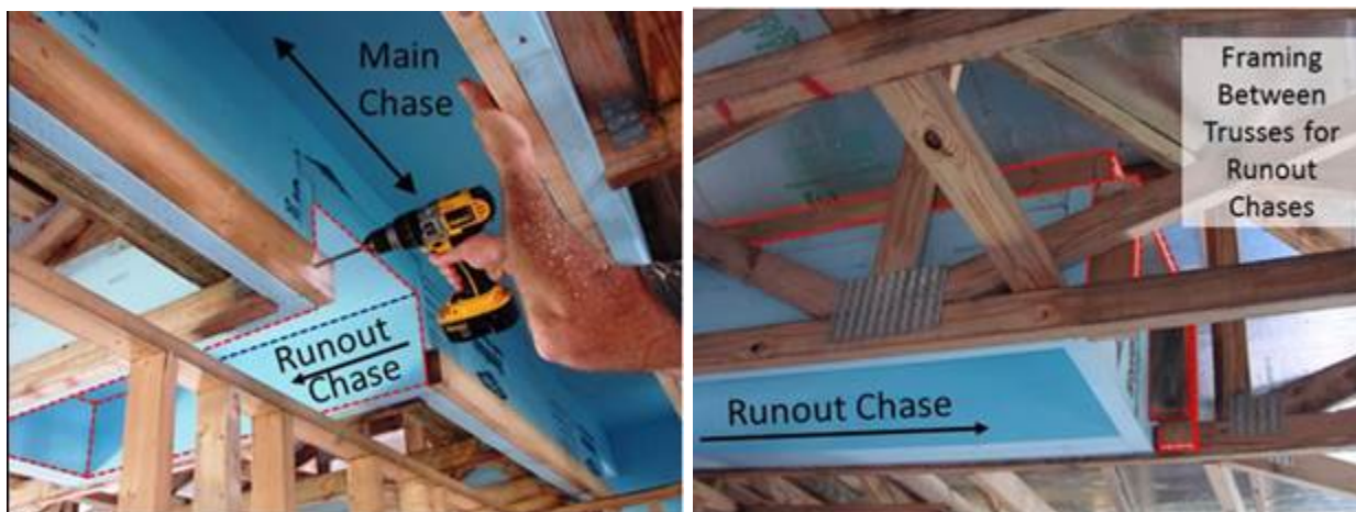
Figure 28. Runout chases seen from underneath (left) and the attic (right). Note dead wood framing between trusses that provides attachment surfaces for the foam air barrier.
