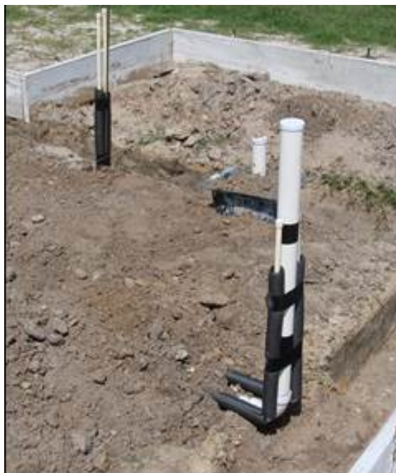
Figure 7. Insulated pipes under the slab foundation
