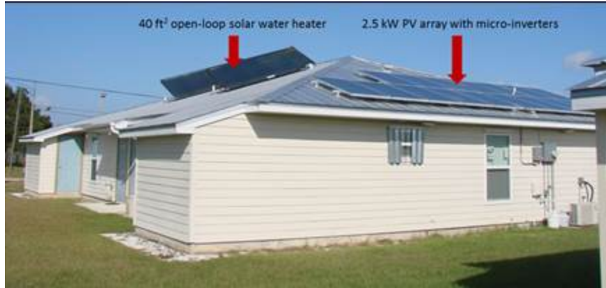
Figure 9. Solar thermal and solar PV panels
