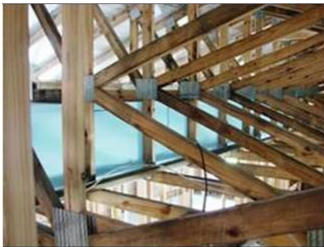
Figure 21. SEVHFH duct chase created using a modified truss design, seen here from the attic side
