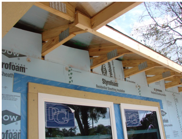
Figure 24. SEVHFH exterior wall primary drainage plane formed by donated Dow Styrofoam rigid insulation
