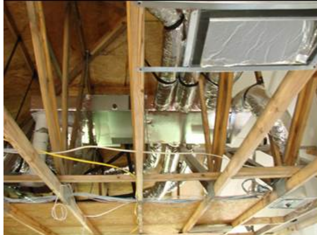
Figure 6. Mechanical system in unvented attic formed by open-cell spray foam (not yet installed) under roof decking
