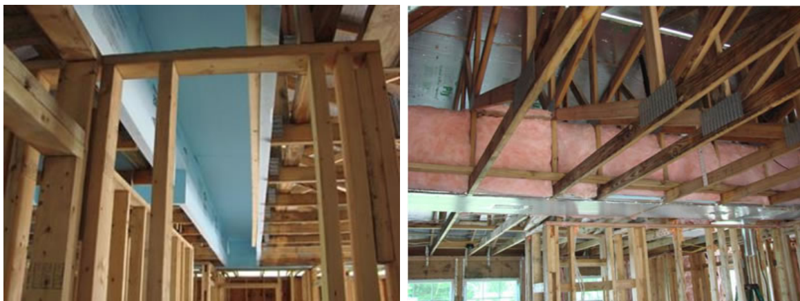
Figure 25. SEVHFH fur-up duct chase with a double layer of 2-in. blue board insulation (R-20 total) (left) and R-13 attic-side fiberglass batt insulation (right)
