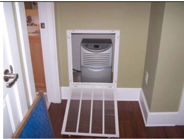
Figure 7. The stand alone dehumidifier is located in the return air plenum.
