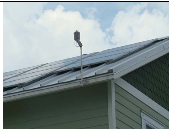
Figure 9. A weather station on the roof line records ambient data.
