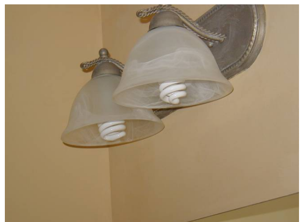
Figure 3: Compact fluorescent lighting is installed throughout the house.
