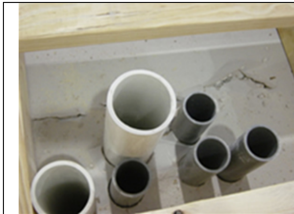
Figure 8. FSEC installed chases in the factory to facilitate wiring for the PV and data acquisition system.
