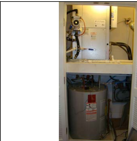
Figure 6. The geothermal unit and water heater share the same mechanical closet.
