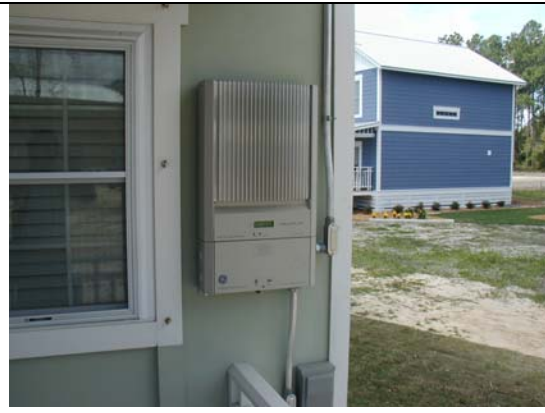
Figure 13. The inverter is mounted on an exterior wall inside the home's front porch.
