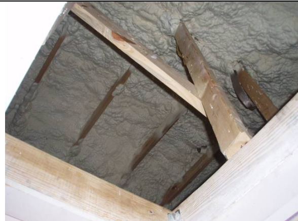
Figure 5. Foam insulation is applied in the attic and in the crawlspace after the home arrives on site.
