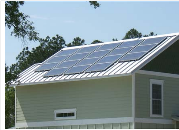
Figure 12. Close up of the 3.6 kW PV system.
