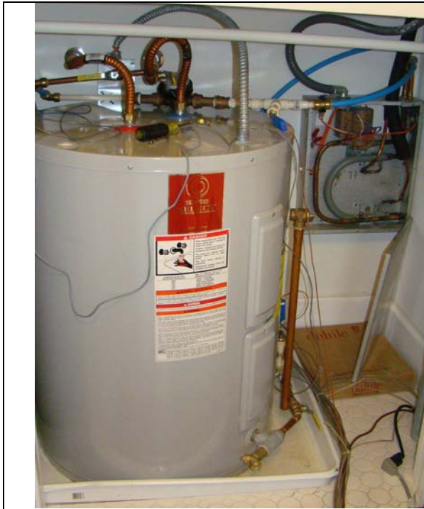
Figure 16. The desuperheater and hot water tank are adjacent to each other and below the geothermal unit.
