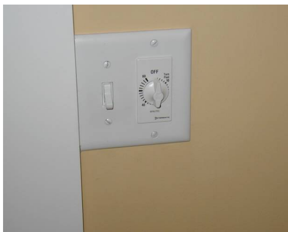
Figure 2: Energy Star bathroom exhaust fans are operated on timer switches.
