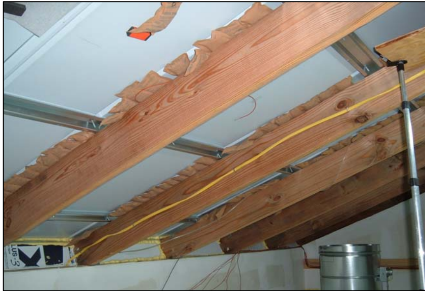
Figure 3. Interior Detail of Experimental NightCool Sealed Attic with Exposed Metal Roofing on Metal
