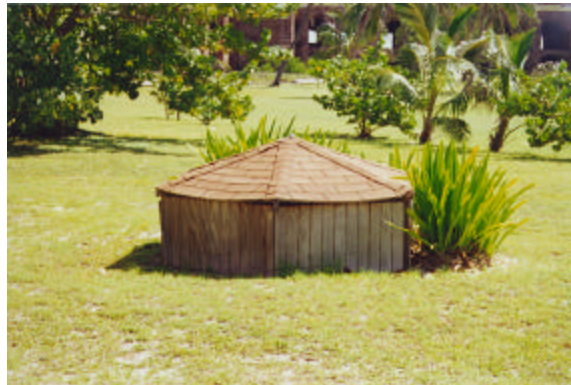
Figure 12. Sewage lift station located in parade grounds.
