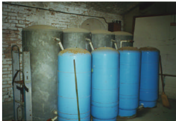
Figure 11. Freshwater and seawater bladder tanks.
