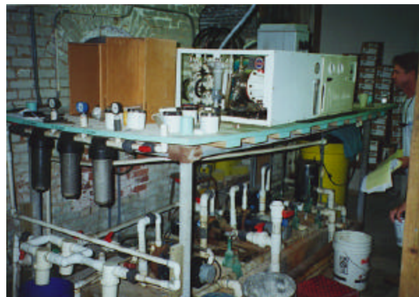
Figure 7. Reverse osmosis system, freshwater and seawater pumps.
