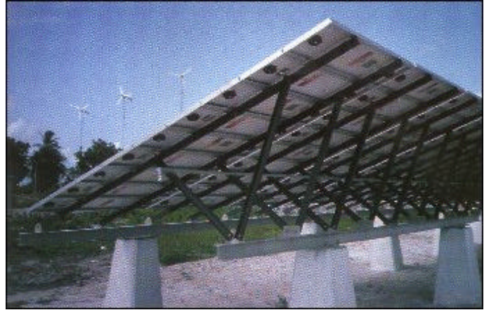
Figure 27. PV - wind hybrid system (SSI).
