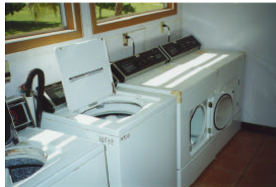
Figure 17. Conventional washers and LP gas dryers.
