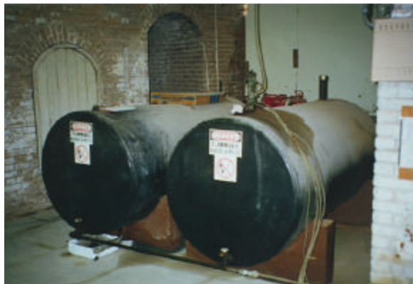
Figure 4. Intermediate diesel tanks.
