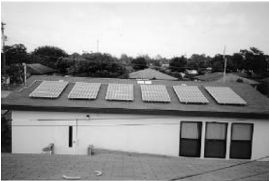
Figure 4. Picture of a utility-interactive PV system on a portable classroom in Lakeland, FL
