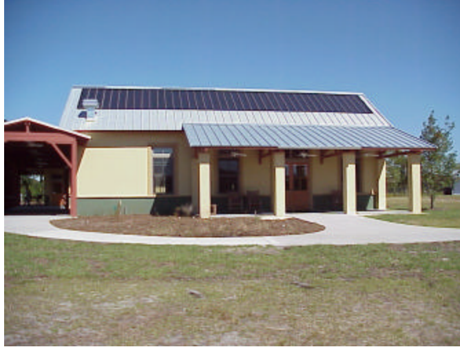
Figure 5. System #2 photovoltaic array.
