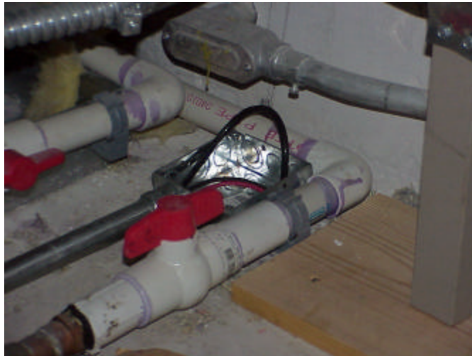
Figure 11. Wiring from inverter to distribution panel, System #2.
