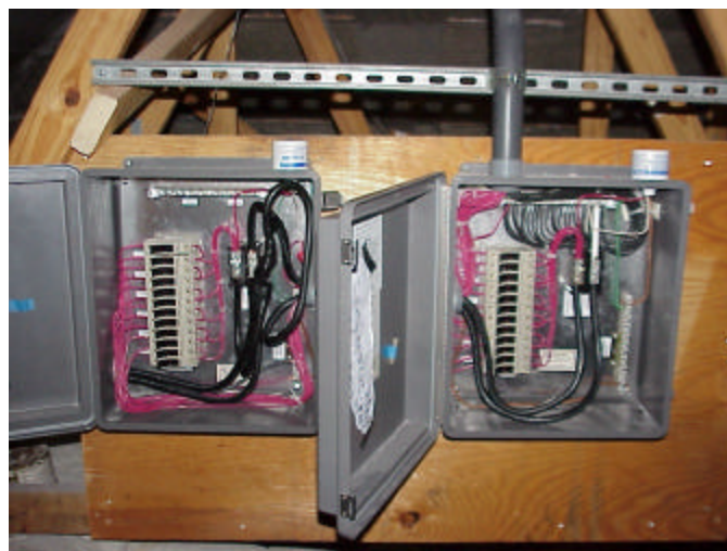
Figure 3. Source circuit combiner boxes for System #1.
