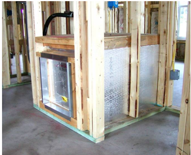
A Ducted return air plenum pulls air only form the conditioned space - not form connected floors, walls, or ceilings. Note frame for filter back grill
