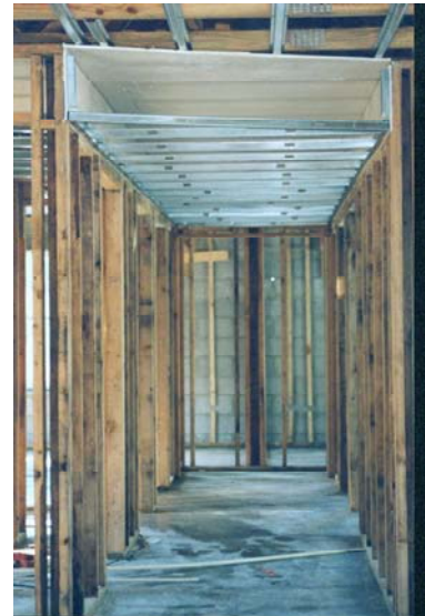
Interior duct chase for supply ducts separated from the attic by a dry wall air barrier
