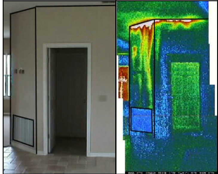
Figure 2. Thermograph of air being drawn from the attic to the air handler in a Florida house.
