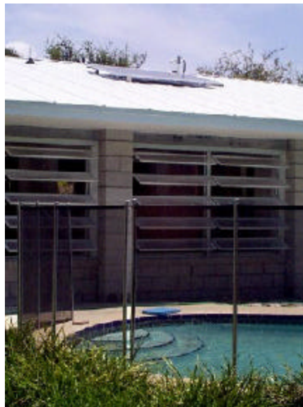
Figure 4. PV array mounted on a white metal roof for pool pumping
