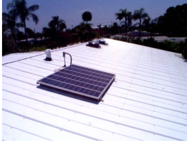
Figure 2. Standoff-mounted PV array on a metal roof
