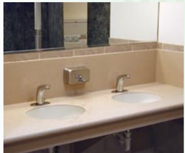
Figure 21. Automatic faucets limit the length of time water flows during one activation, thereby ensuring flow is not left on.
