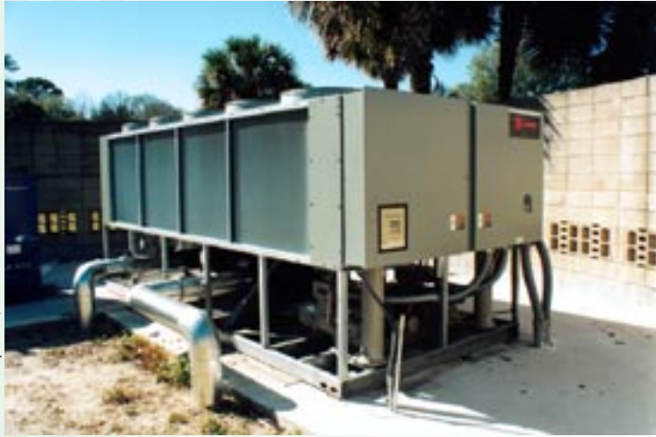
Figure 20. Heating and cooling system maintenance needs to be performed regularly to maintain equipment life and occupant comfort.
