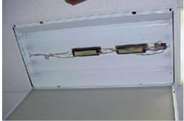
Figure 11. The fixture is stripped of its lamps.
