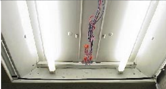
Figure 12. Two T-8 lamps are used in place of the four T-12 lamps, and recentered.
