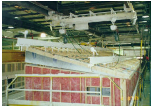
Figure 12. Installing all or part of a photovoltaic system on manufactured buildings in a factory environment may significantly reduce non-module costs and provide greater quality control.
