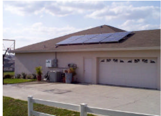
Figure 3. A residential PV system in Lakeland, Florida that is typical in size and design to those proposed for distributed generation experiments.
