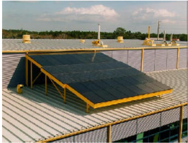
Figure 6. This 12-kW PV system is designed to withstand a category 3 hurricane.
