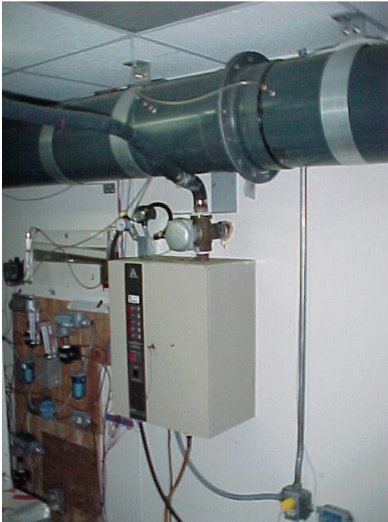
Figure 3. Steam Generator and Airflow Station
