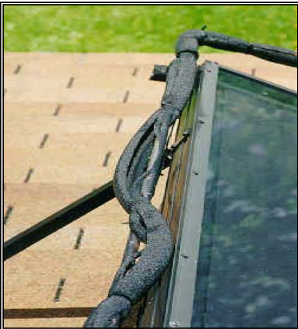
Figure 6.3-10a. Plastic-based insulation should not be used for exterior piping.
