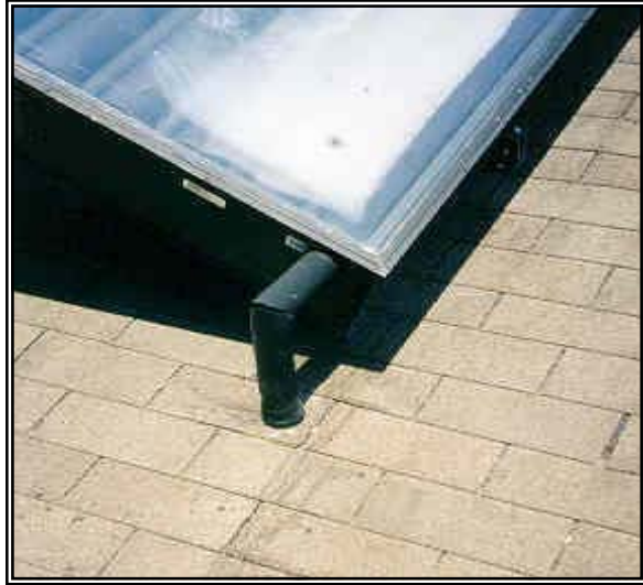
Figure 6.3-11b. Use of 45 degree angle cut and insulation glue provides a positive and aesthetic seal.
