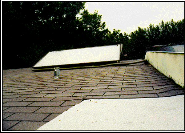
Figure 6.3-5a. Collector return line can not be completely drained due to upswing in piping. At times, this is unavoidable due to the layout of the roof and access locations.
