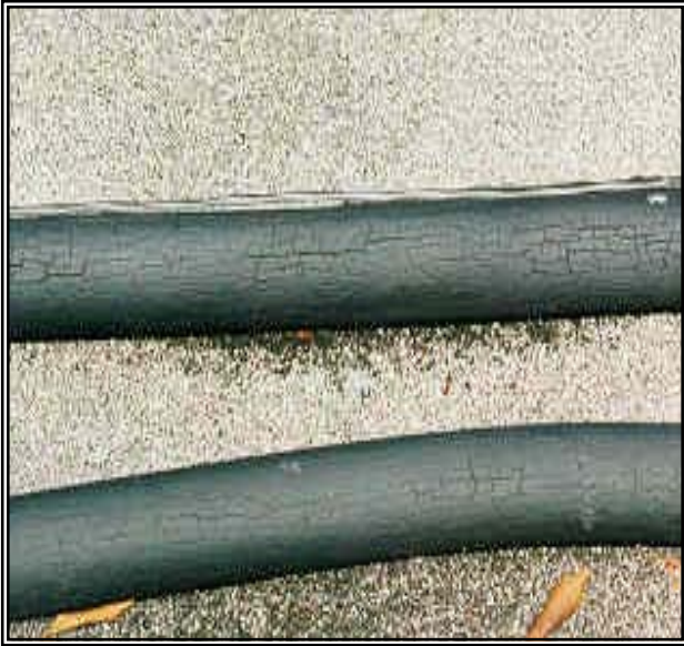
Figure 6.3-9a. Cracking and eventual deterioration will occur if insulation is not ultraviolet ray
