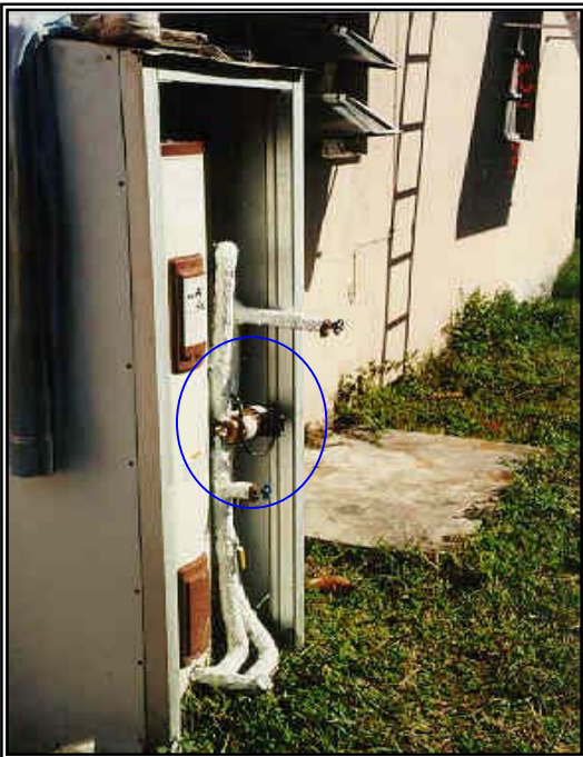
Figure 6.3-18a. Top and sides of water heater protected, but not front. Pump is exposed to elements.
