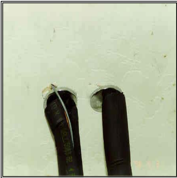
Figure 6.3-21a. Ceiling penetration left bare.
