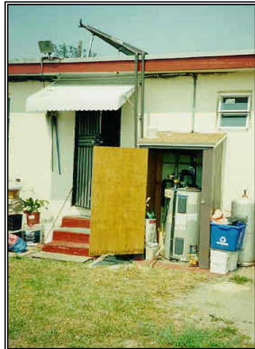
Figure 6.3-18b. Water heater and components enclosed in storage shed.
