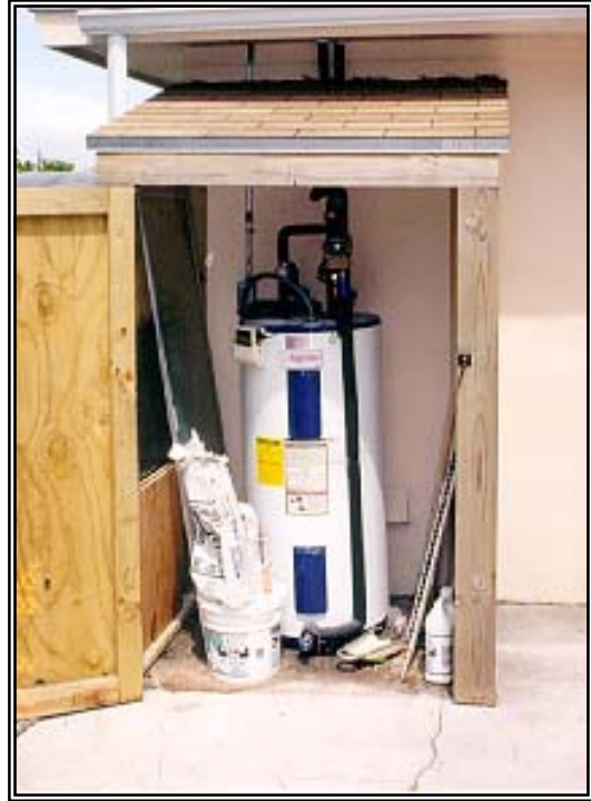
Figure 6.3-19b. Solar pump and controller are protected.
