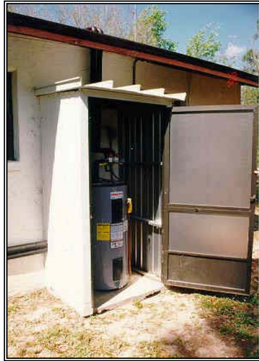
Figure 6.3-20b. Protected water heater and solar components.
