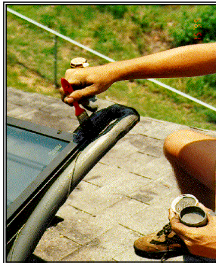
Figure 6.3-8b. Care is taken to make sure that all exposed piping and sensor wires are ultraviolet ray protected.
