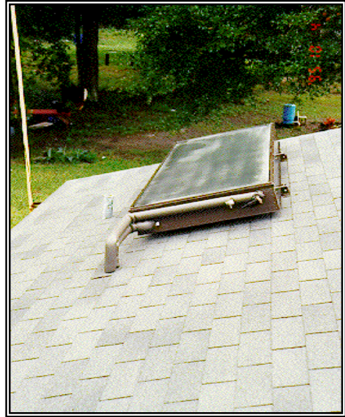
Figure 6.3-9b. Well protected insulation will last many years.
