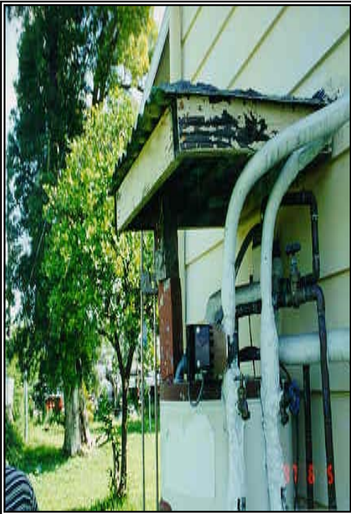
Figure 6.3-20a. Minimal water heater and component protection.
