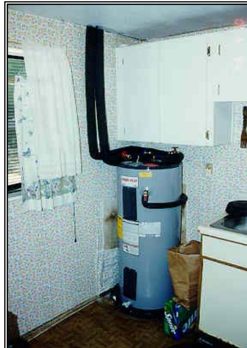
Figure 6.3-22b. Neat solar plumbing and insulation installation to water heater.
