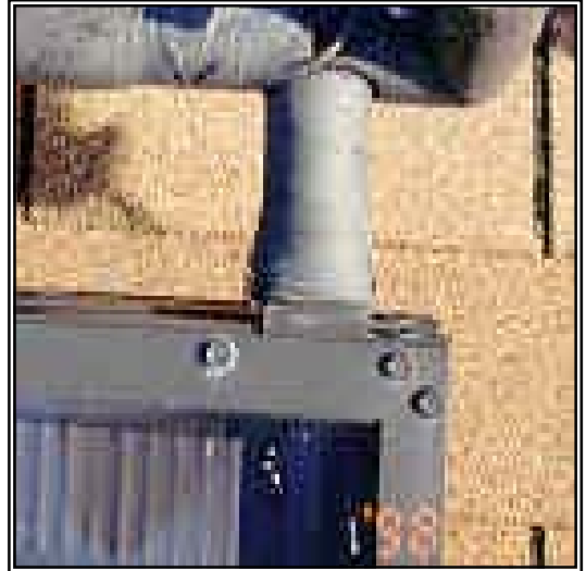
Figure 6.3-13b. Collector sensor is secure and protected from environmental conditions.
