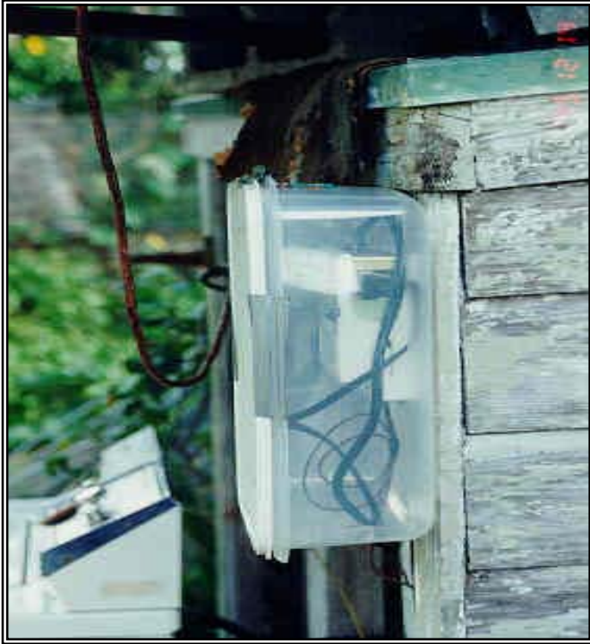
Figure 6.3-19a. System controller protected by common Tupperware enclosure.
