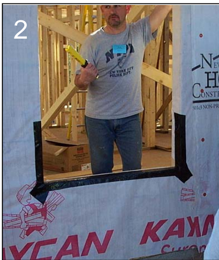
2 Sill flashing with wide flashing tape. (Alt: adhesive back membrane, pre-formed pan flashing, felt.)
