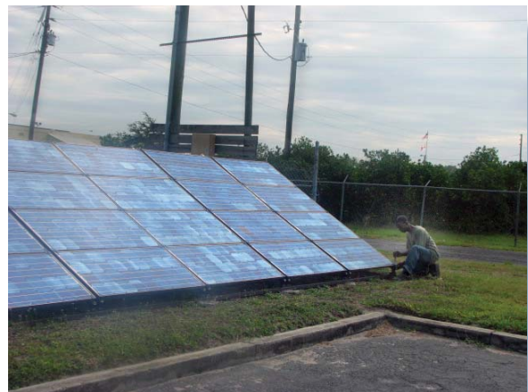
This photovoltaic system at Westside Tech is one of four on campus generating solar electricity for the school.
