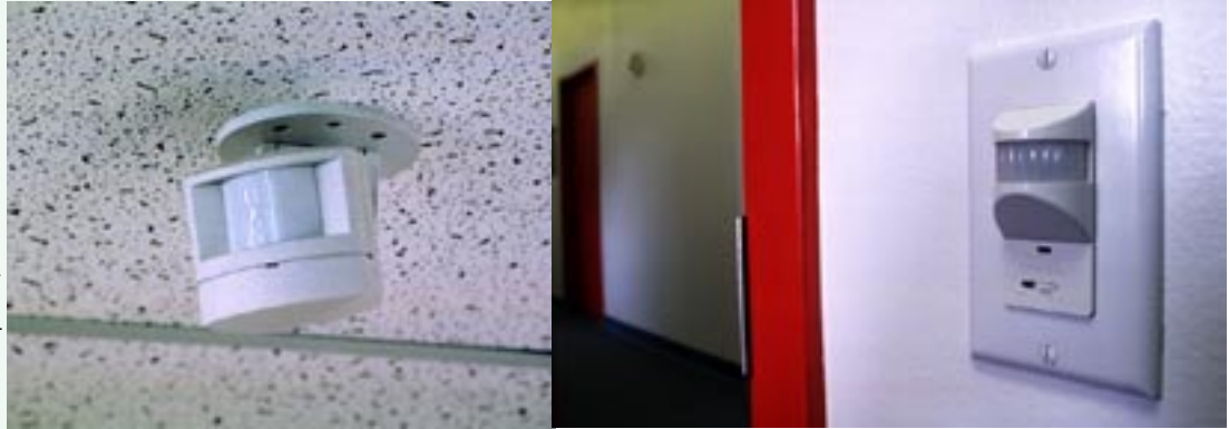
Figure 15. Two examples of infrared motion sensors. The one on the left is a ceiling mount, and the one on the right is a wall mount.
