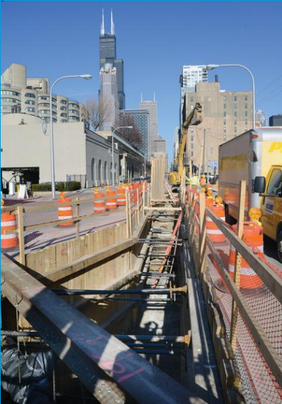
Source: ComEd Underground 345kV Project
