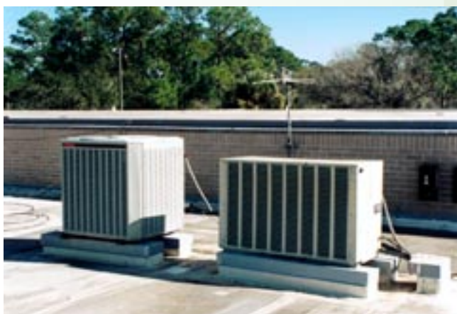
Figure 5. Flat roofs like this one are prone to water accumulation.
