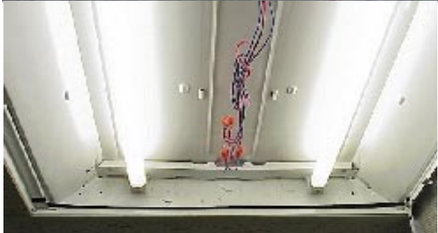
Figure 12. Two T-8 lamps are used in place of the four T-12 lamps, and recentered.
