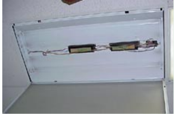
Figure 11. The fixture is stripped of its lamps.
