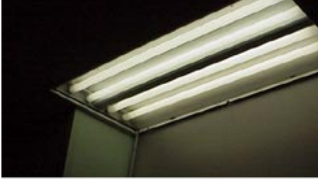
Figure 10. In this example, a fixture containing four T-12 lamps is slated for delamping.
